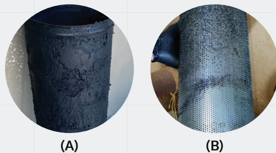
Figure 1. SWD Inlet Filter (A) before Verza application and (B) after Verza application.
