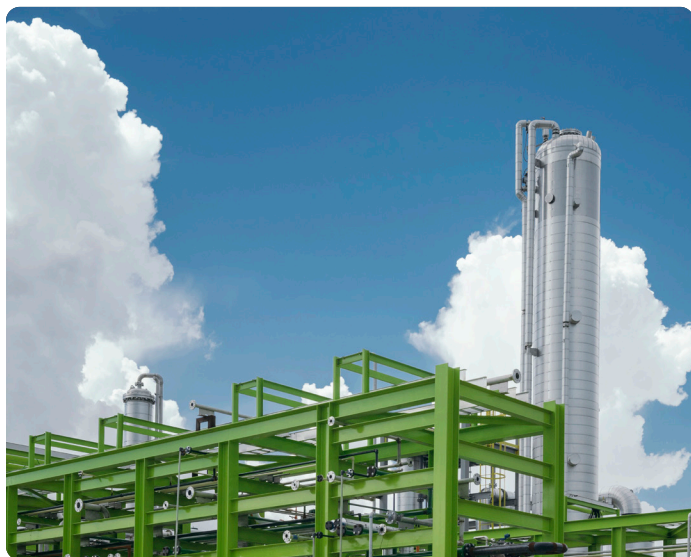
Solugen's first-of-its-kind Bioforge plant in Houston, TX.
